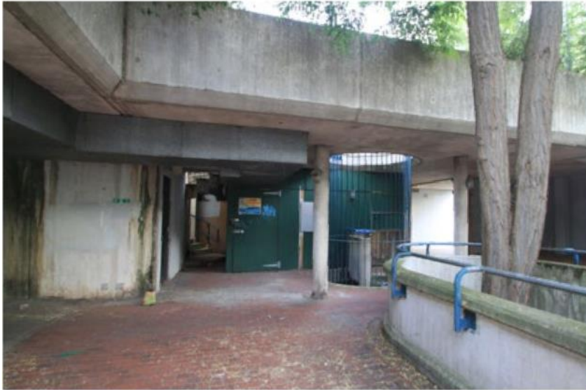
Existing ductwork fixed to soffit of walkway, connecting boiler room to block A5
